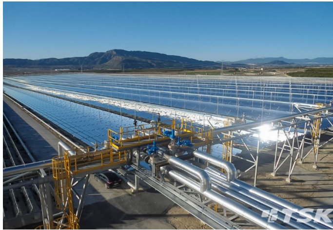
Figura 8: Central termosolar Fresnel puerto errado 2 Fuente: http://www.cspfocus.cn/en/study/detail_93.htm
